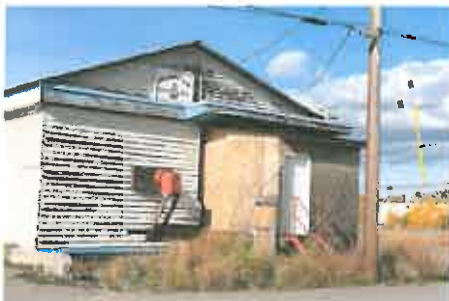
Uncared for buildings convey a negative message and reflect poorly on the area they are in. This entrance is as visible as the front door.
