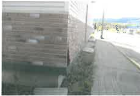
Low quality or inauthentic building materials and poor workmanship do not age well and quickly fall into disrepair reflecting poorly on the area they are in.
